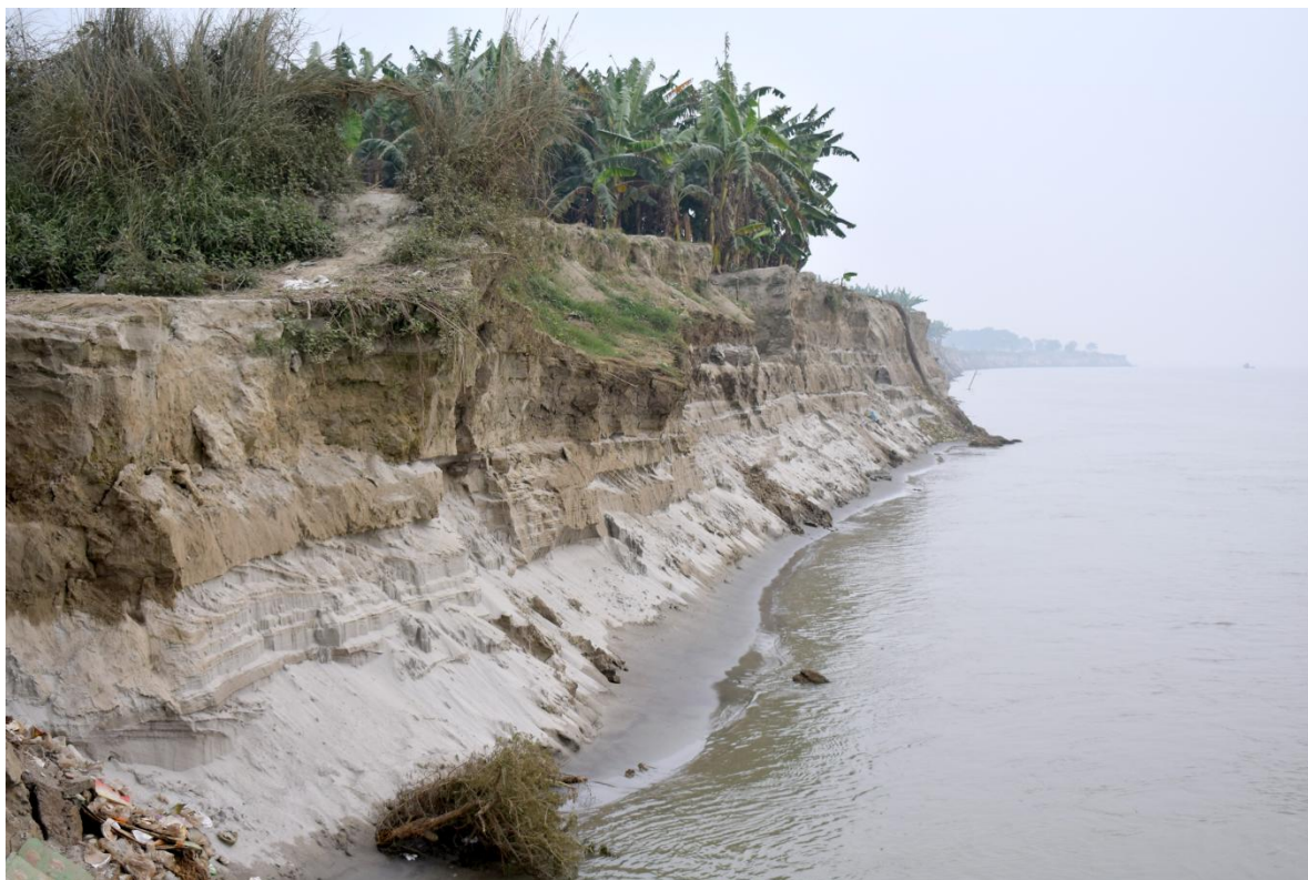
Image 43 : Lateral Bank Erosion Observed Near Maniarpur In Vaishali Distt.
